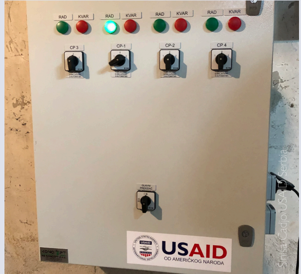
JKP Čačak SCADA Control Panel
