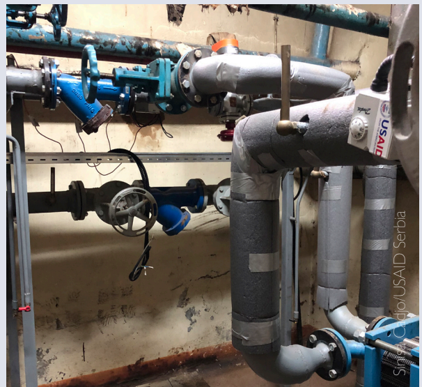
JKP Čačak SCADA Temperature Sensors
