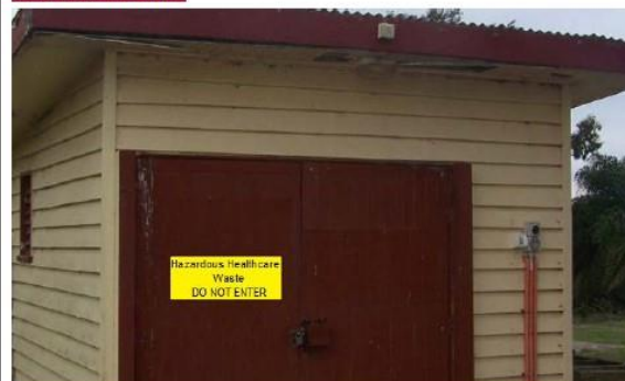
Hazardous healthcare waste storage room observed with appropriate signage, working locks, and adequate space for waste storage prior to offsite transport.
