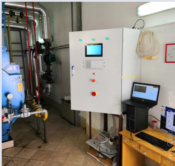
Automation system at Ratko Jović
