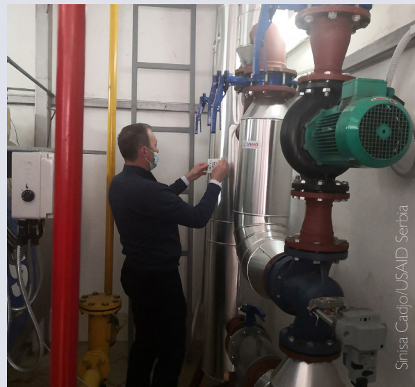
Temperature sensors and ancillary equipment at Majakovski
