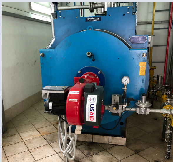
New burner (in red) at the DHC Niš Ratko Jović substation
