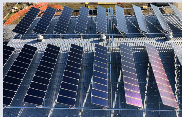
The JKP Grejanje roof-mounted solar thermal system on the Kotež boiler house.
