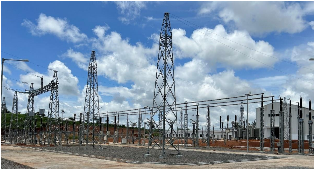
An electrical substation in Kamakwie, Sierra Leone; part of the CLSG interconnection line. Photo Credit: Power Africa
