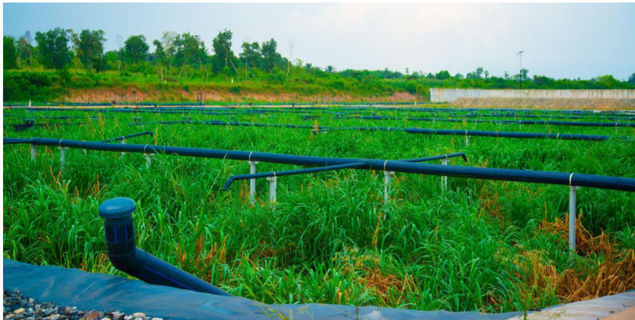
Abomey-Calavi FSTP's sludge disposal channel and buffer tank. Photo Credit: MuniWASH
