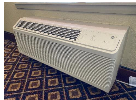
Figure 6. Room Air Conditioner
