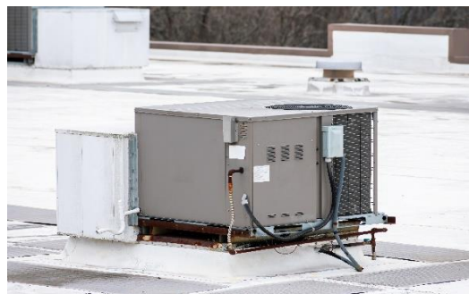
Figure 9. Packaged Rooftop Unit
