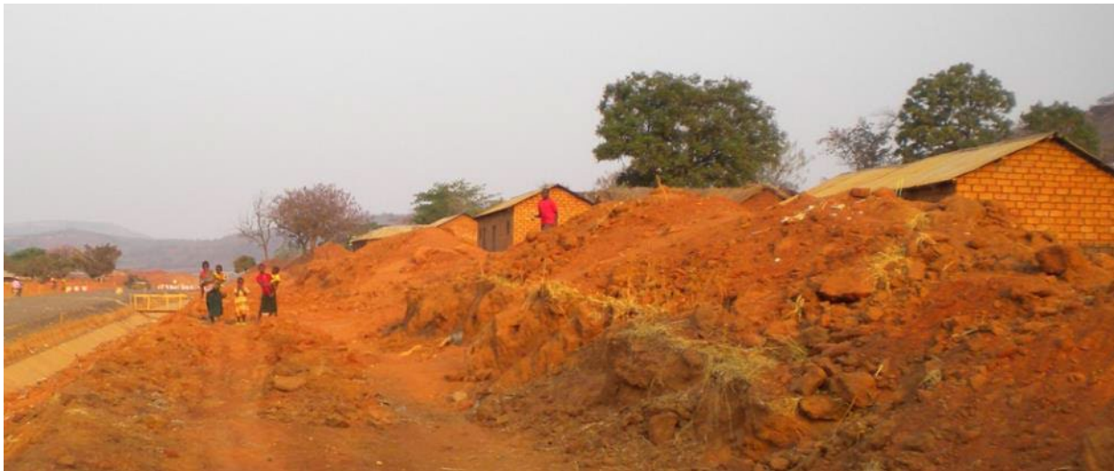
Figure 23. Temporary Spoil Piles Blocking Access to Homes
