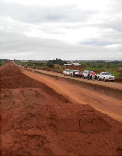
Figure 25. Exposed Soil During Construction
