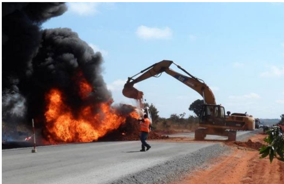
Figure 37. Bitumen Truck on Fire
