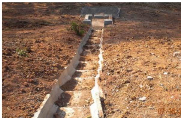
Figure 30. Stepped Drainage Channel
