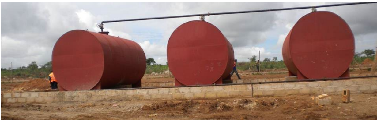
Figure 5. Fuel Storage Tanks with Bund Wall
