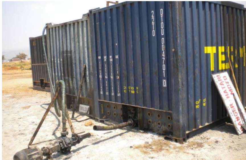
Figure 21. Heated Containers for Bulk Bitumen
