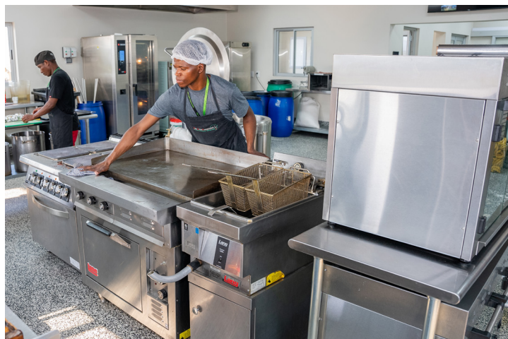
TLC staff member cleaning an electric grill and twin-basket fryer obtained through LEPP. Photo credit:TLC
