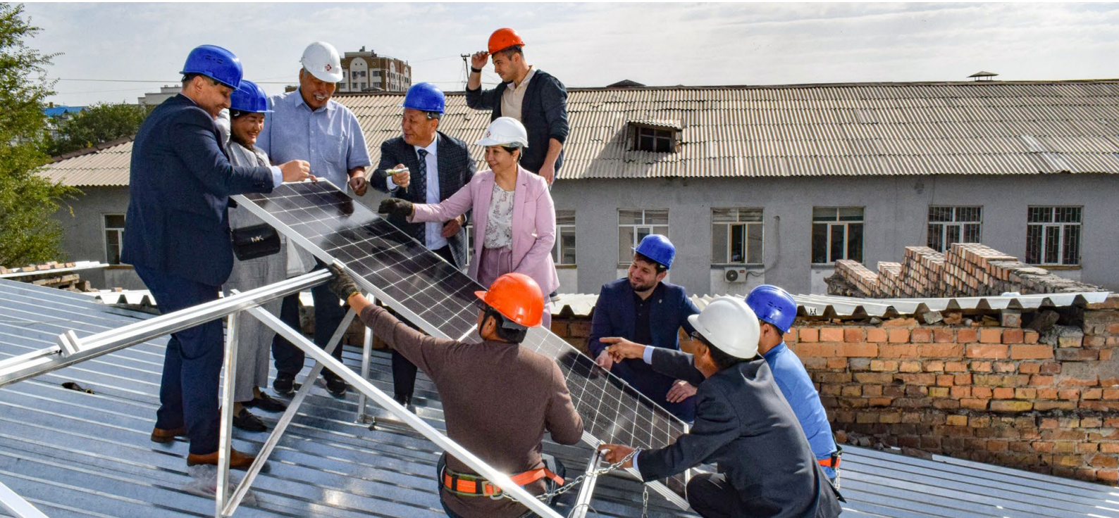
PHOTO: THE USAID POWER CENTRAL ASIA ACTIVITY
