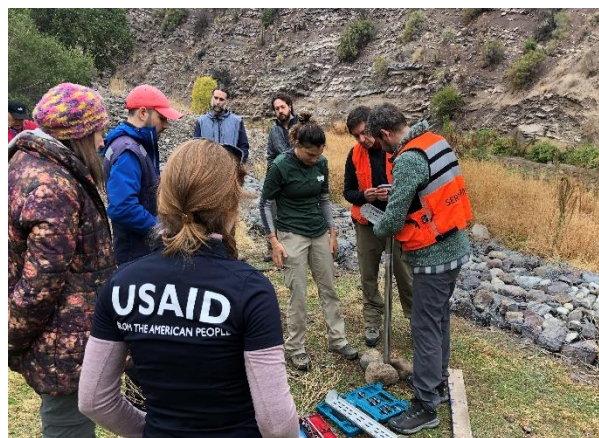
USGS scientist advises geological scientists from the Government of Chile on the installation of a landslide monitoring station beside the Maipo River basin near Chile's capital city of Santiago. Photo courtesy of USGS and Stephen Slaughter.
