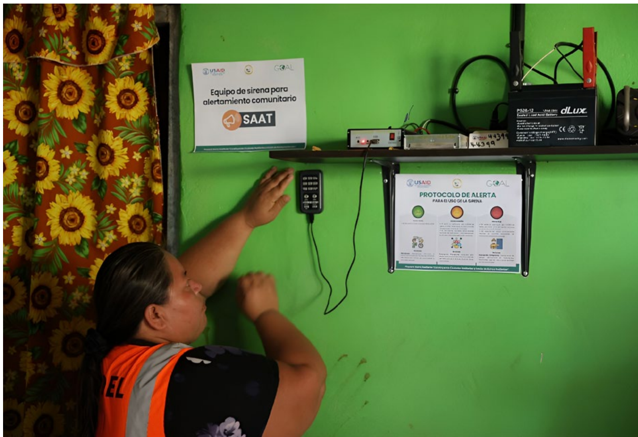
USAID helped develop a new early warning system in Villanueva, Honduras, to make the community more resilient to natural hazards, such as flooding and landslides. Photo: Dakota Gardner/USAID.
